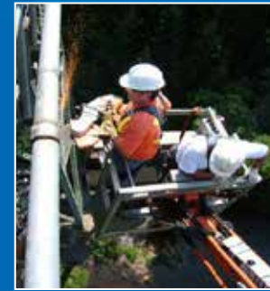
TELECOM NETWORK MAINTENANCE
