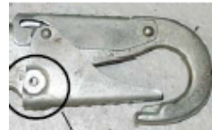
Broken / Missing Rivet
